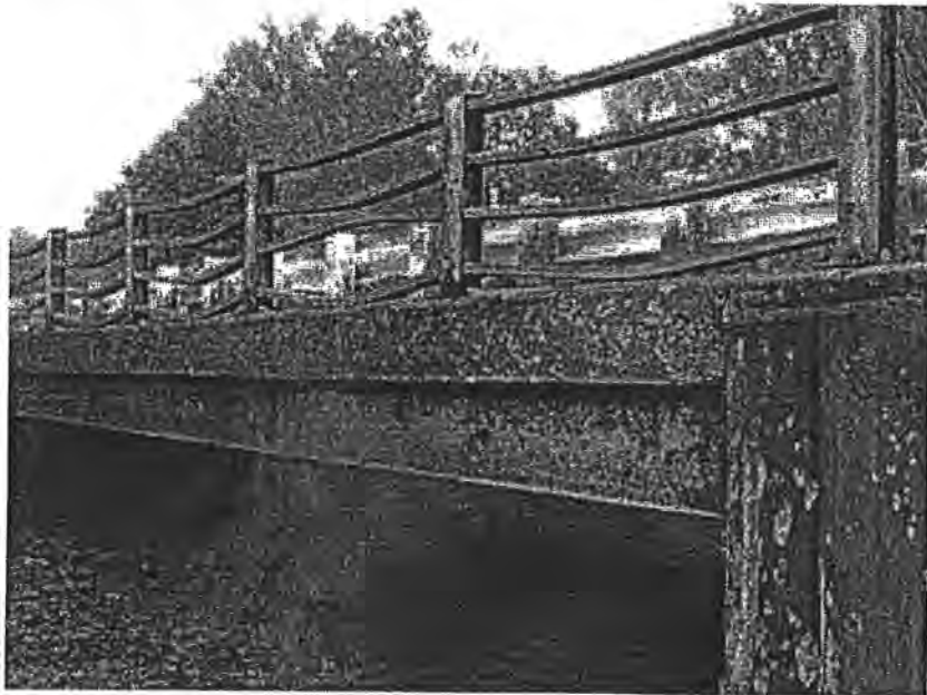
Figure 6.13 Facia of fire damaged bridge
